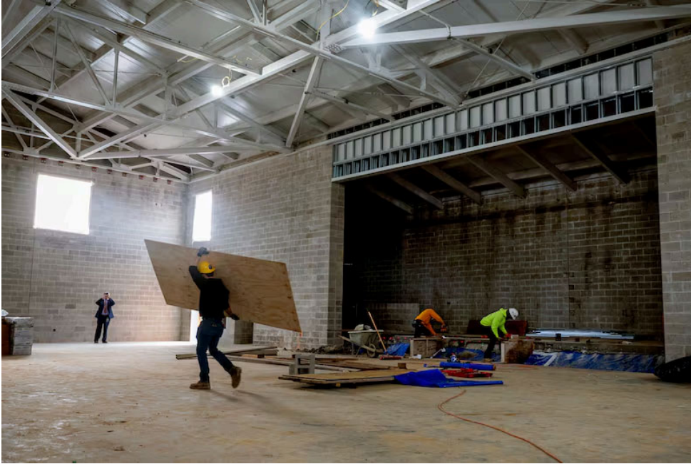
Construction is underway on a new all-purpose room at Joseph D. Sharp Elementary School in Cherry Hill. The work is funded by a $363 million bond referendum approved by the district's voters in 2022. Tom Gralish / Staff Photographer
