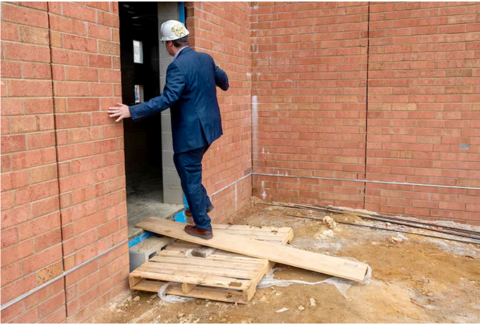
Principal Ric Miscioscia enters the construction site to get his first look in a few months at the progress of the new all-purpose room and gym at Joseph D. Sharp Elementary School in Cherry Hill last Read more Tom Gralish / Staff Photographer
